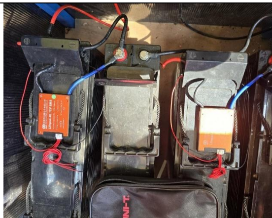
Percobaan pengujian charging baterai 2 x 12 V tipe VRLA
